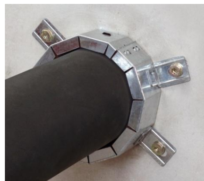
Caption - correctly installed pipe penetration
