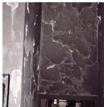
Flame spread over painted surface
