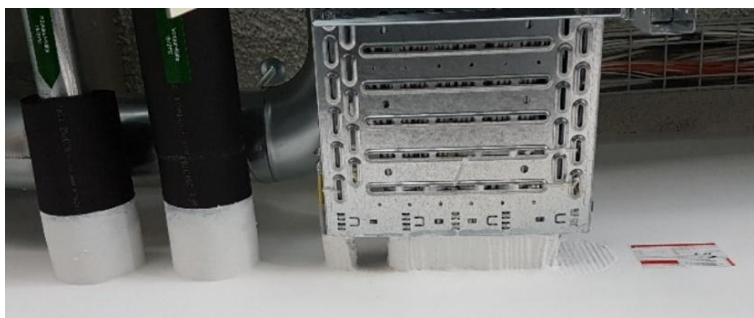
Installed cable and pipe penetration seals
