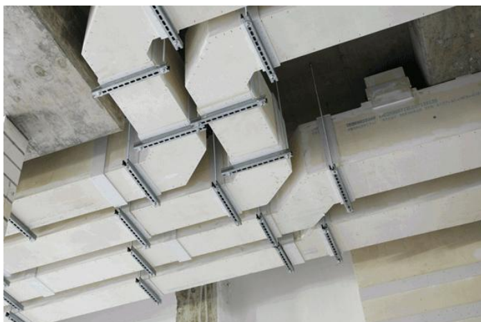
Fire resisting ducts
