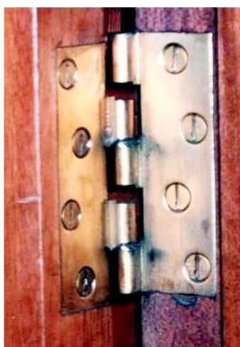
Worn hinges allow the door to drop
